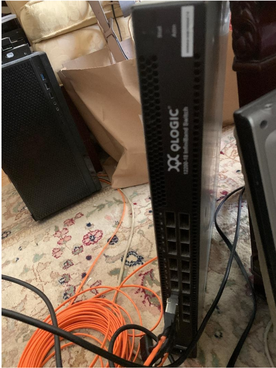
Figure. 1.1.7 [High Performance Switch (HPS) Network Switch Qlogic]
